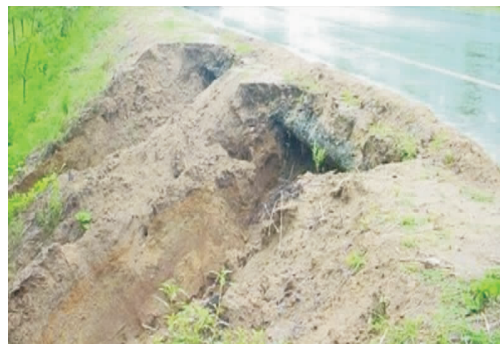
(c) 边坡冲刷
